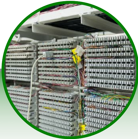
Telephone central office
